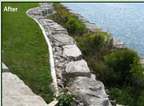
Completed in 2010, steel sheet wall was replaced along the Guthrie Park shoreline with armour stone and native vegetation, providing habitat for fish, birds and insects. Small mammals, such as muskrat and mink, are already using the easier river access for foraging and hunting.
